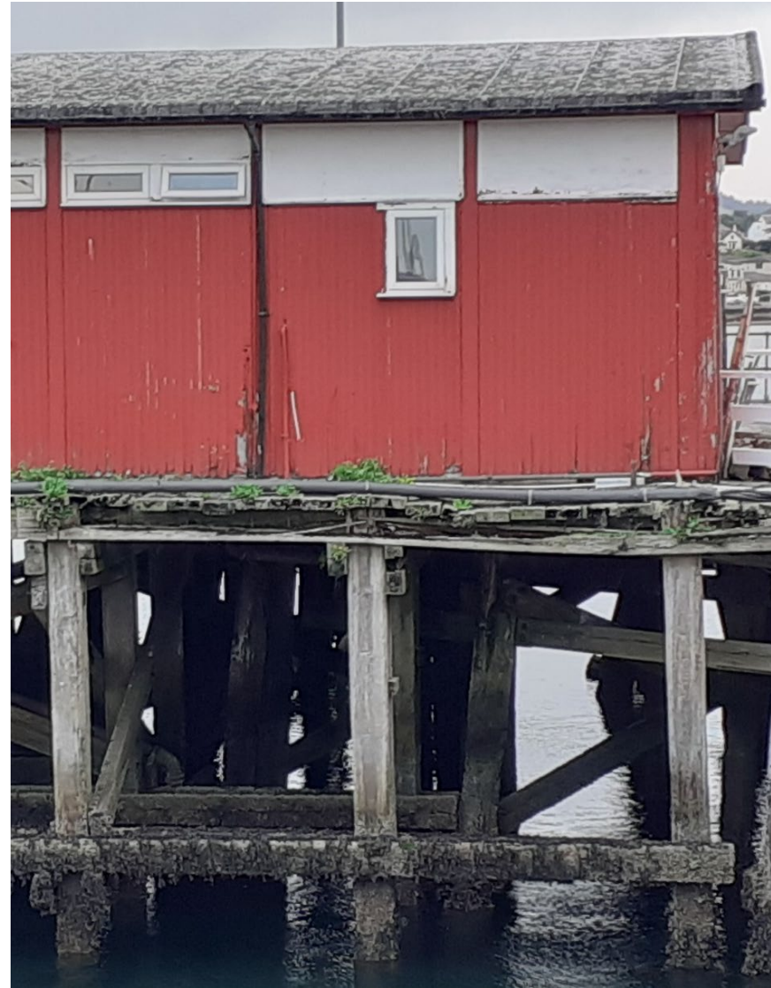
Image B2.2 Victorian Pier, deteriorated decking
